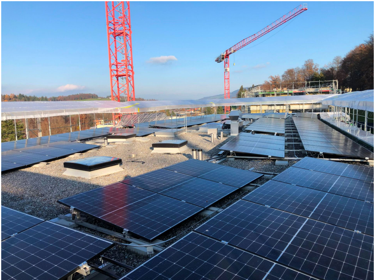
Figure 5: Typical collector field (photo by the manufacturer)
